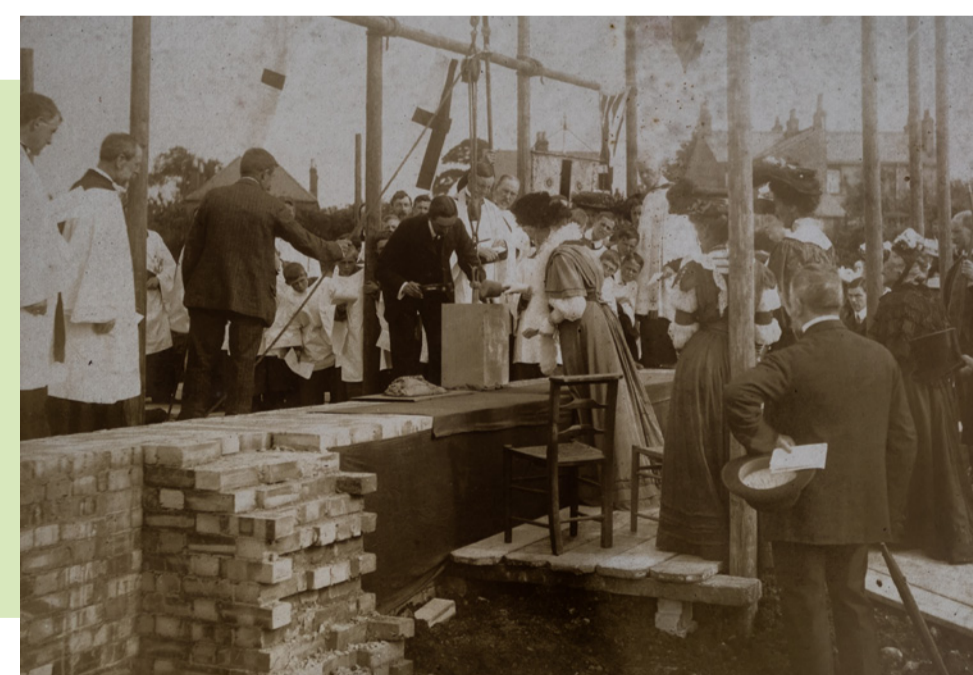
Black and white photograph of St John’s being built. Laying of the foundation stone by Mrs Tylston Hodgson, 27 th July 1907.
